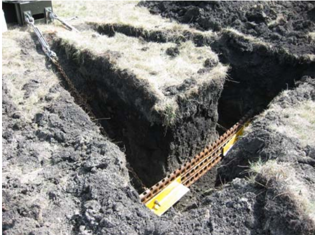
Ground Anchor for Temporary Barrier
